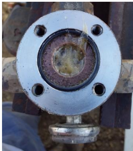
Figure 4 Valve clogged with thick foam concentrate.
